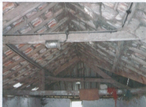
Fig. 5: Roof of the preparatory shed with no outlet and subsequent poor ventilation, demonstrated by lots of cobwebs.
