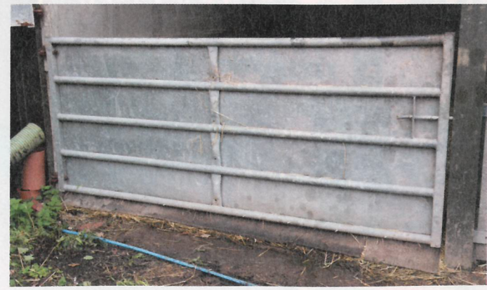
Old conveyor belts are fixed to the bottom of gates to prevent badger access.
